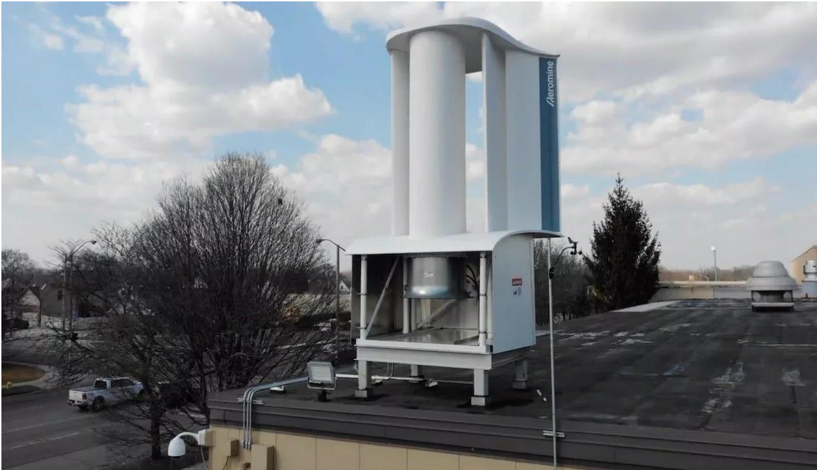
The Aeromine rooftop wind device. Aeromine Technologies
